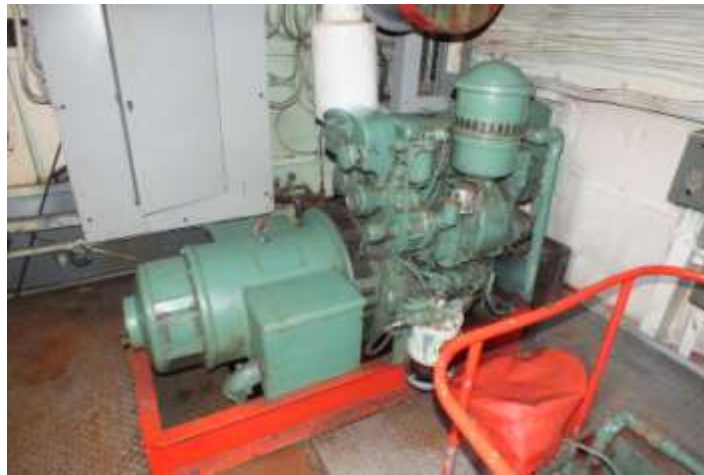
Port main generator.
