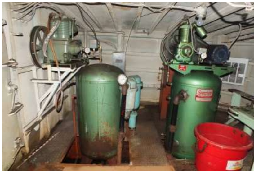
Pair of SPEEDAIRE compressors and storage tanks in lazarette.
