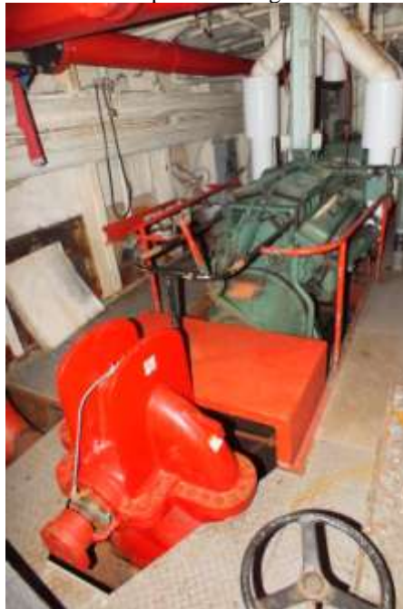
Port main drive engine, PTO and fire pump.
