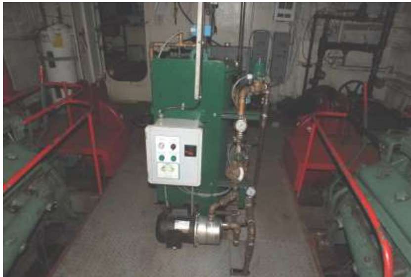
BOSS system in Engineerroom.
