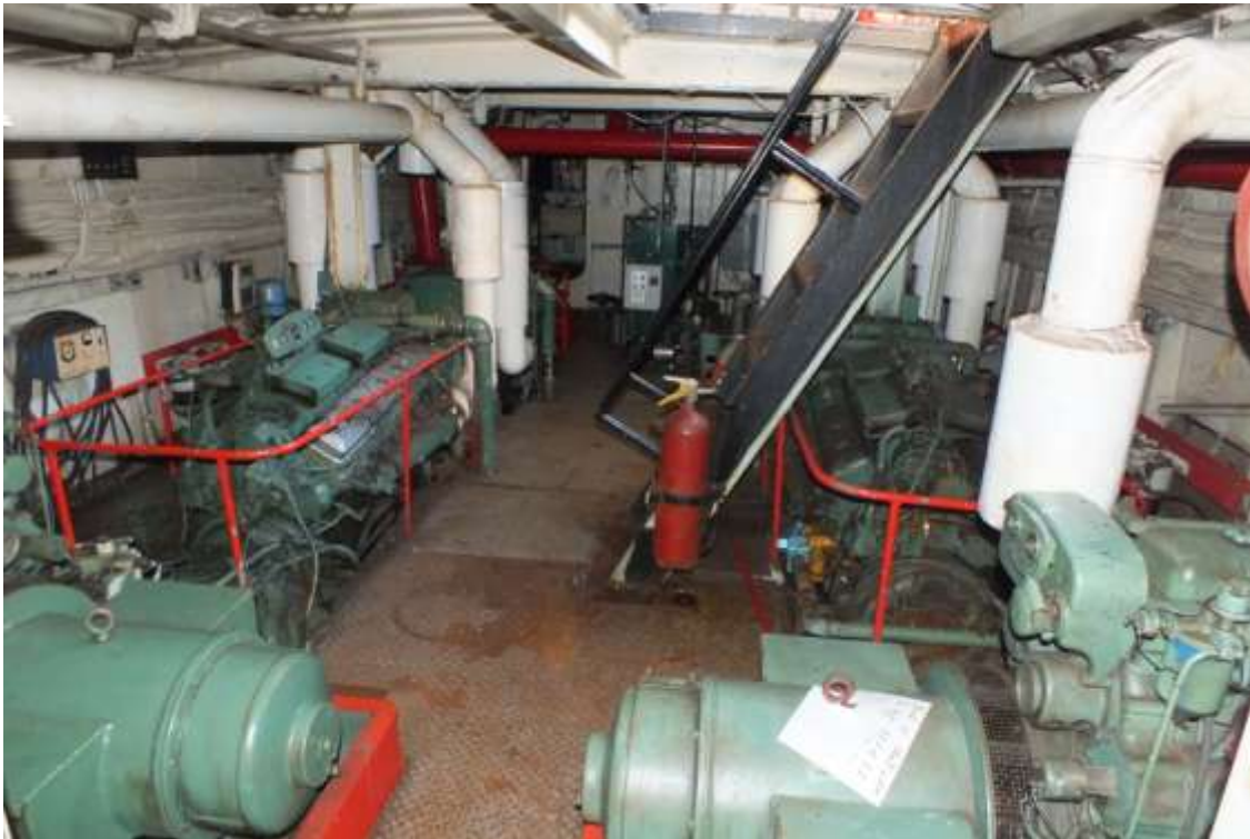
Engineroom, looking forward.
