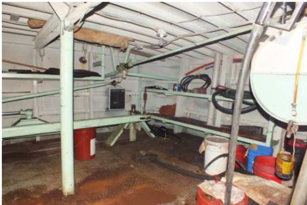
Port side of lazarette, showing lube oil tank and port steering/rudder post assembly.
