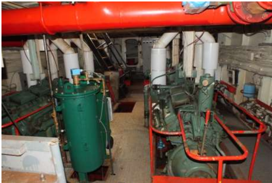
Engineroom, looking aft.
