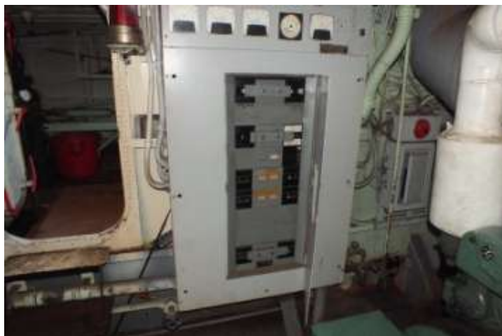
Main genset control panel
